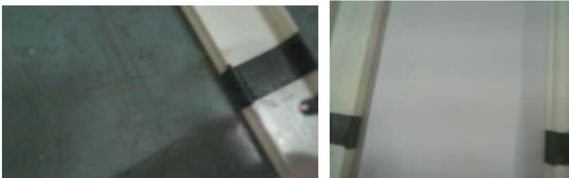
Fig 5.4: ESP32-CAM Captured Image of Crack
