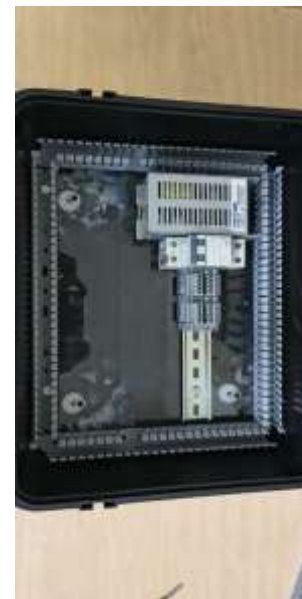
Fig. 4. Internal power and control section (MCB, 24 V DC SMPS, terminals and integrated controller on DIN rail).
